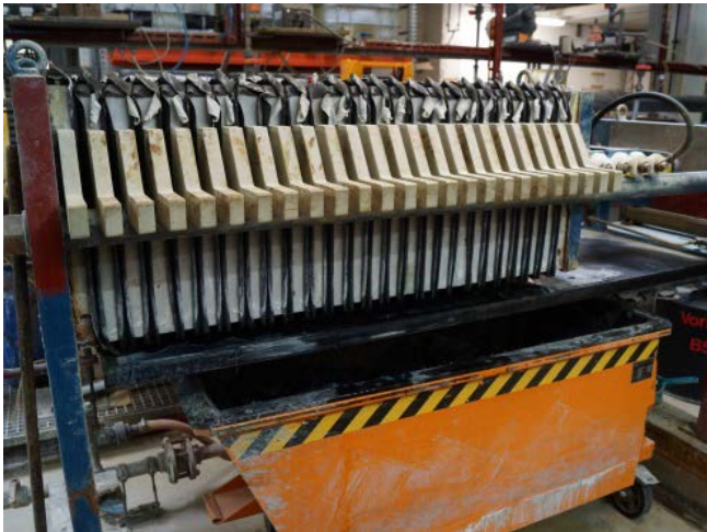
Photograph shows filter press for dewatering solids on wastewater treatment plant.
