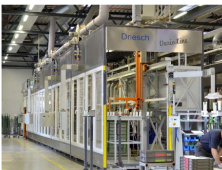
Photographs show chambers enclosing plating systems and hoist lines.
